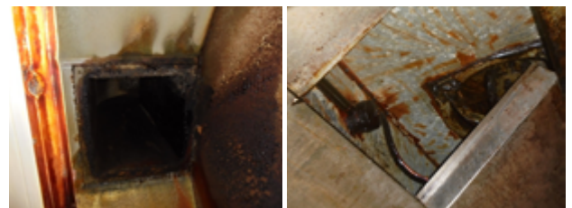
Both photos showing significant build-up of grease residue inside the flues and associated wiring.
