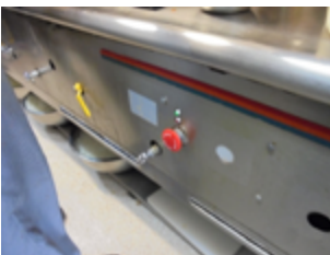
Emergency gas shut-off button and [ball] valve at the cooking appliance
