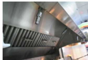
Automatic fire suppression above the deep fryers
