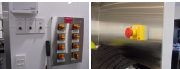
Switches and emergency gas shut-off button on the walls
