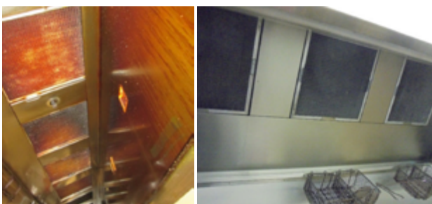
Grease build-up in the filters and hood Clean grease filters
