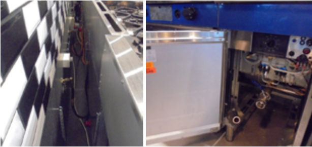
Well-maintained hoses and connectors Clean control panel and mechanical parts
