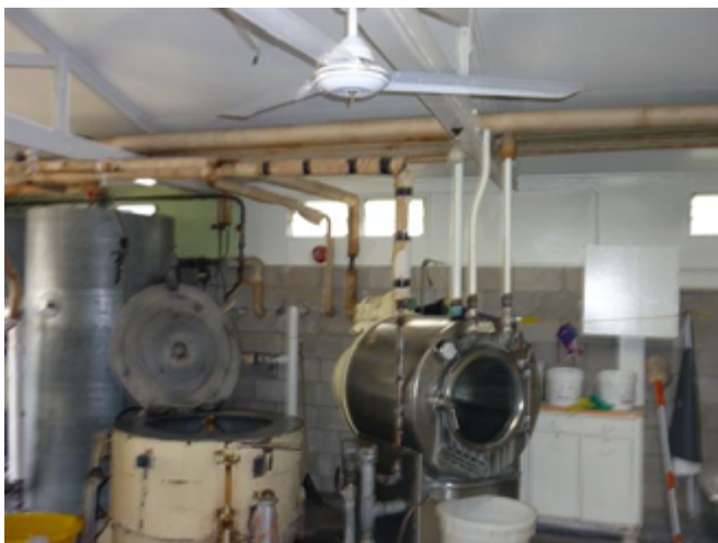
Figure 1 - Gas fired washer and dryer units
